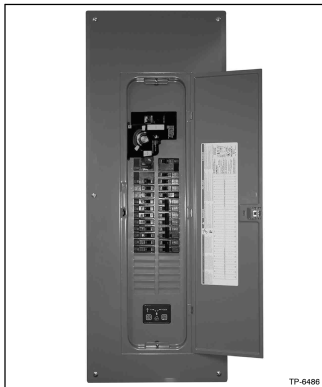
Figure 1 Intelligent Transfer Switch
